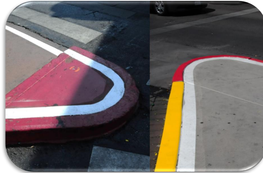
Picture 5.14 – Paint Colors Not in Compliance with MUTCD.
