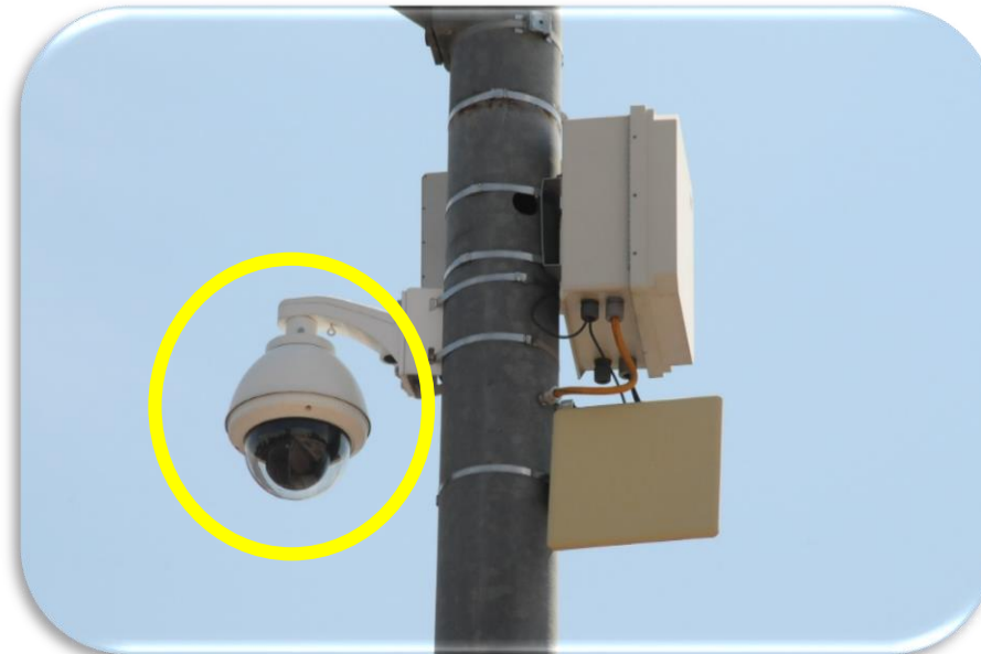
Picture 3.3 – Typical Las Vegas Boulevard Metro Camera.
