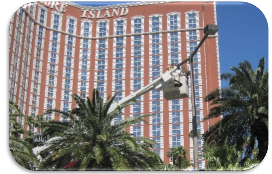
Picture 3.5 – Camera Installation – Treasure Island.
