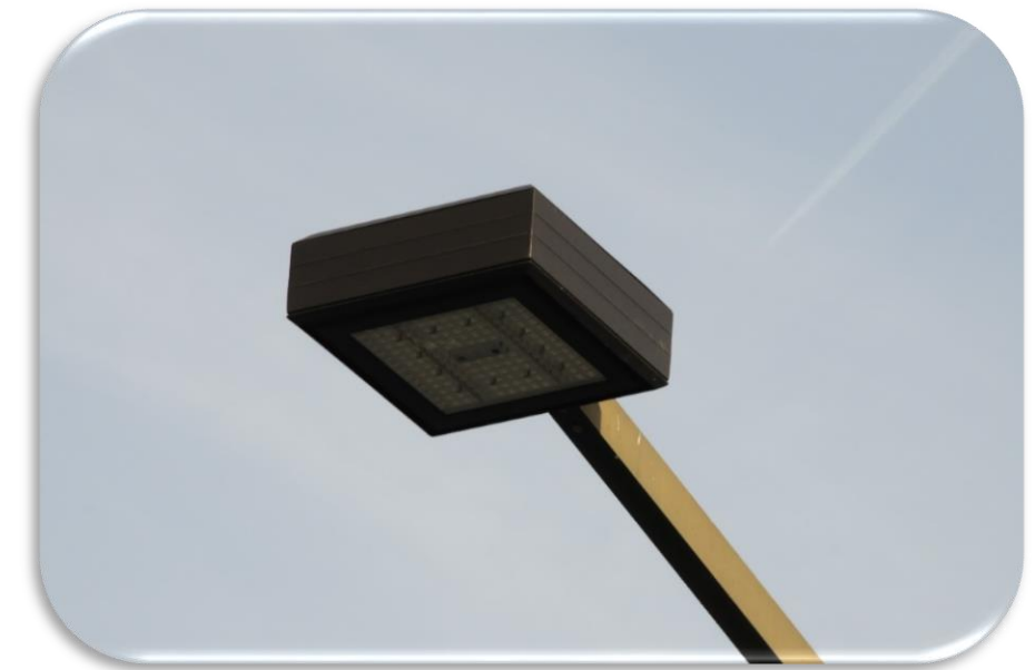
Picture 2.6 – New LED Pedestrian Lighting - 2015.
